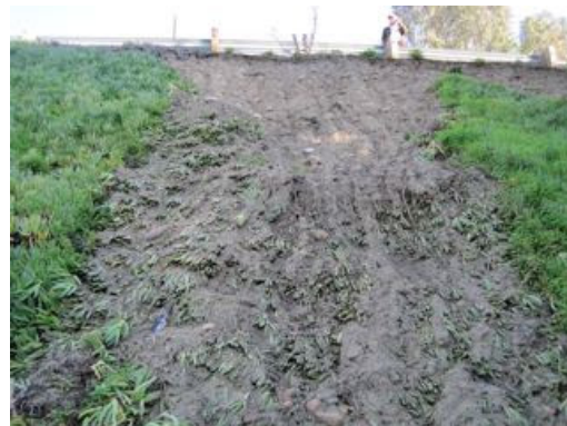
A nasty landslide down a canyon slope covered in non-native iceplant. Photo from www.cnps.org .
